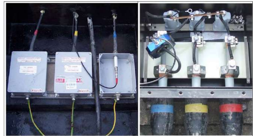
Sensors connection at link boxes
