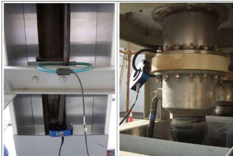
Sensors connection at terminations
