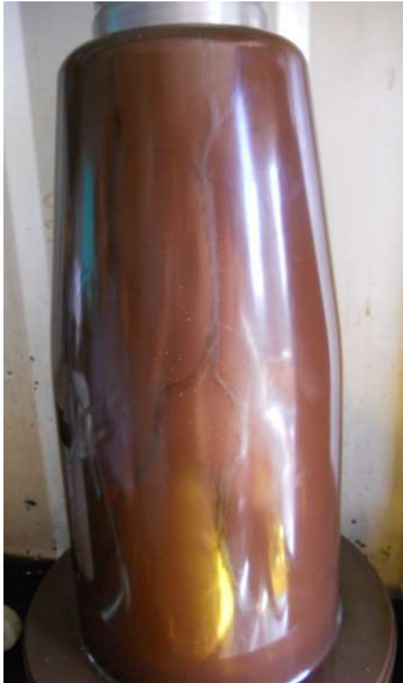
White phase GIS termination disassembled
